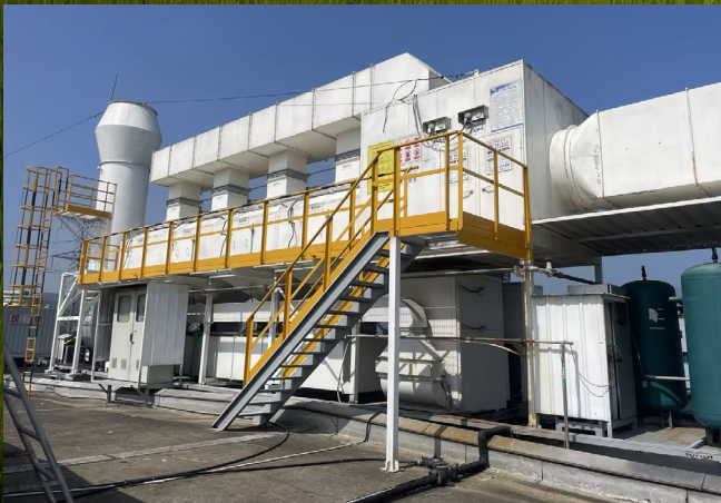
Waste gas treatment equipment
